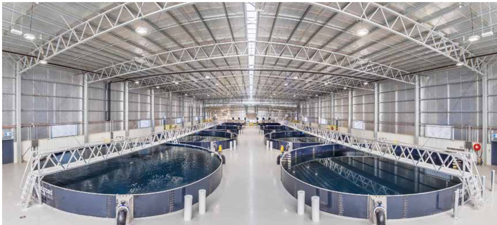
Only part of the 4m deep tanks are visible at ground level – the rest can be accessed via a basement level.
